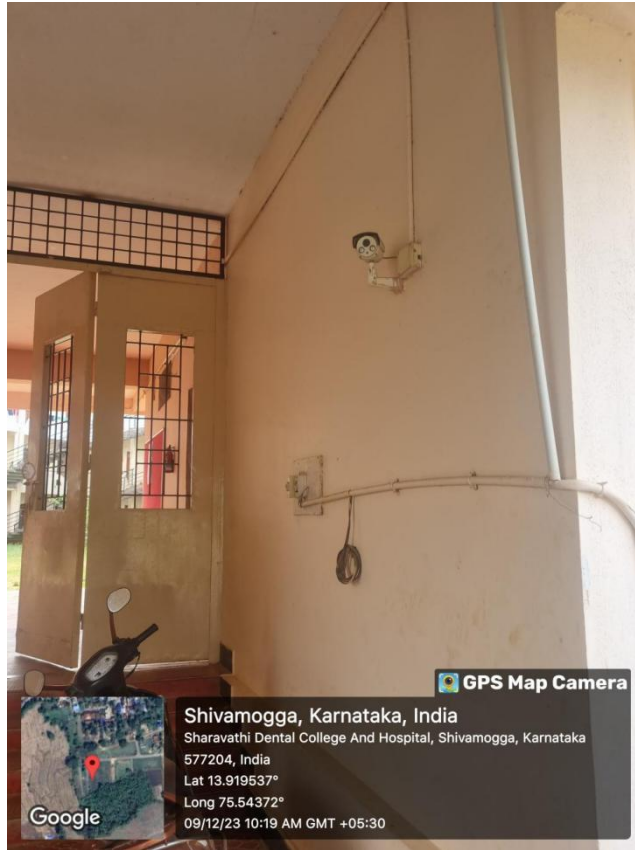
1.CCTV CAMERA OUTSIDE GIRLS HOSTEL ENTRANCE
